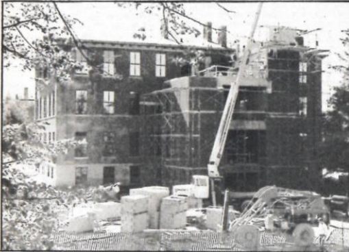
Engel Hall nears completion as the final touches go on the brand new elevator facility. Work on Engle Hall will be finished by the end of October. Across the campus, other construction projects are also in progress. (Photo by Dan Steger)
