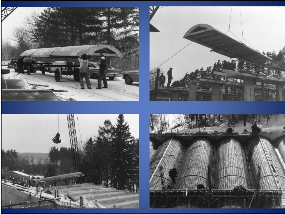
The curved roof segments are put in place, one by one, and coated with cement.
