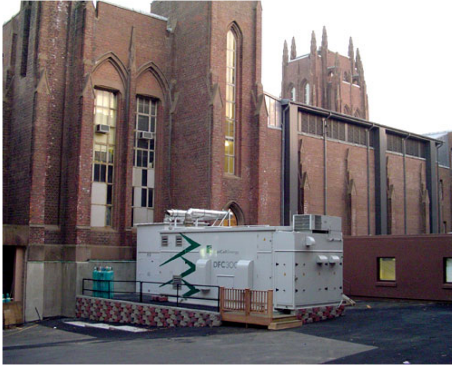
A direct fuel cell from FuelCell Energy installed on the Yale University campus in New Haven, CT.
